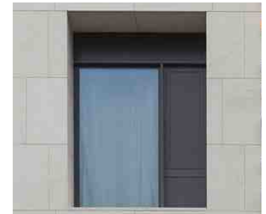
Powder coated aluminium windows with spandrel panels
